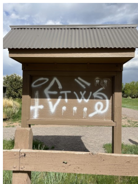
Damaged Hogback Hill Park bulletin board
